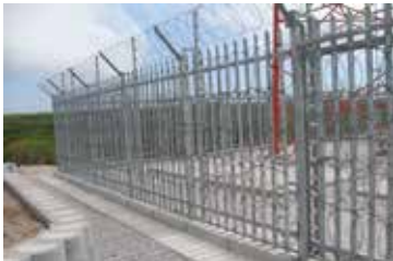
STEEL PALISADE ELECTRIC FENCE
